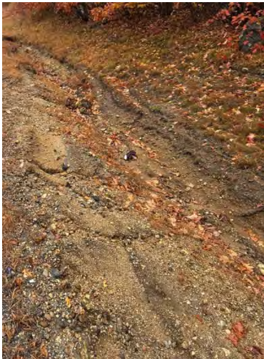
Large erosion gully alongside New Hampshire Route 119. Gully leads to catch basin and stream at the bottom of the hill.
