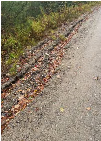
Large gully on side of road.
